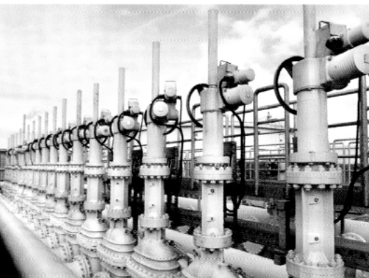
Explosion-proofed actuators mounted on a gate valves.
