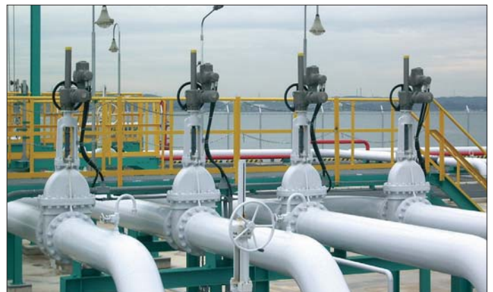
Explosion proof multi-turn actuators SAExC in the kerosene distribution system.
