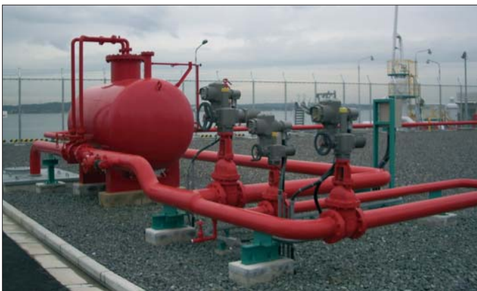
Explosion proof multi-turn actuators have also been specified for the fire fighting system.
